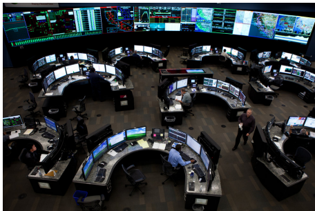
California ISO Control Room
